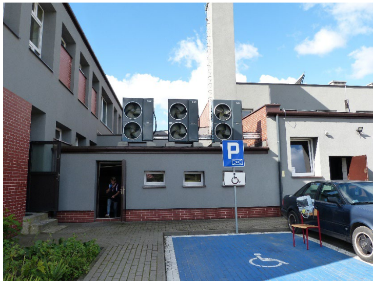
Figure 4 Heat pumps installed in the school roof.
