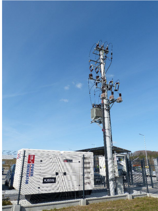
Figure 9 Power generator in the sewage treatment plant.
