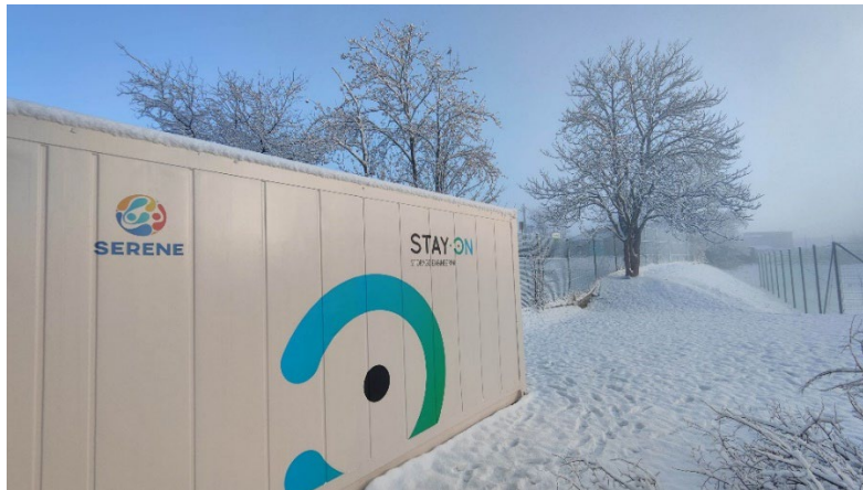
Figure 46 Vanadium Redox Flow Battery container sited next to Arena Przywidz.
